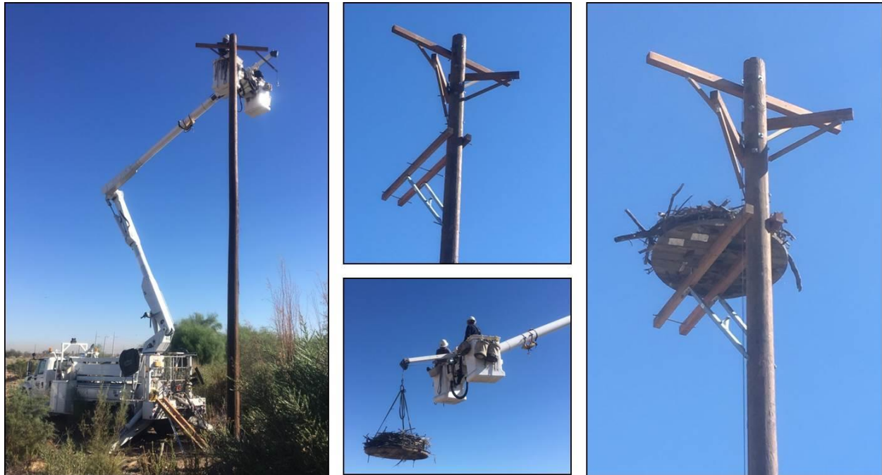
Figure 6. Installation of nest platform (#8) at Pee Posh Wetlands BA on September 29, 2017. Photos by K. McCarty.
